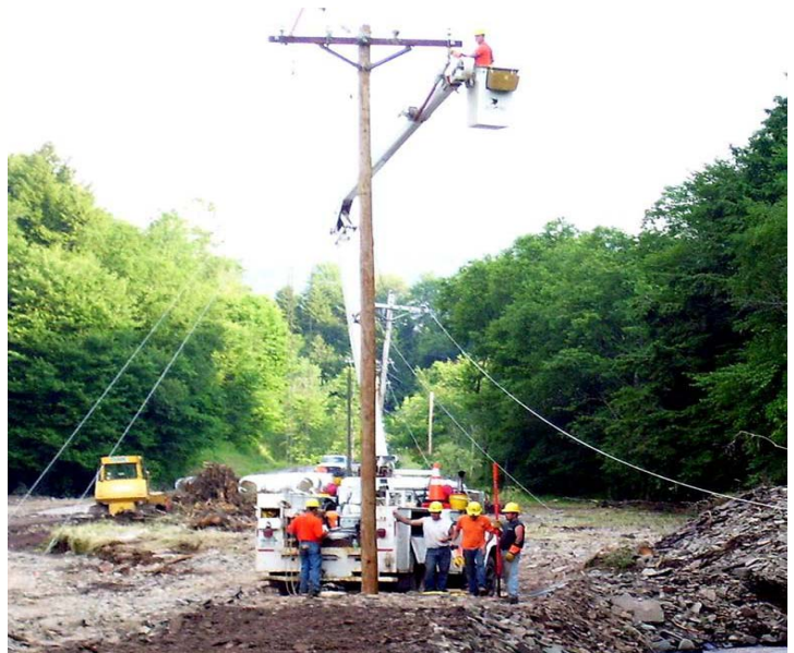
Spring flooding causes significant damage in Delaware County Electric Cooperative crews rebuilding lines after Spring Flood washed away portions of the pole line
